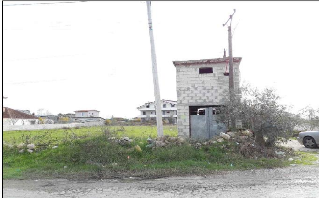
Foto 3: Kabina Murature-Cerme Shkumbin 02-Fideri Nr.4/10KV-N/St Bicukas-Divjake 35/10KV
