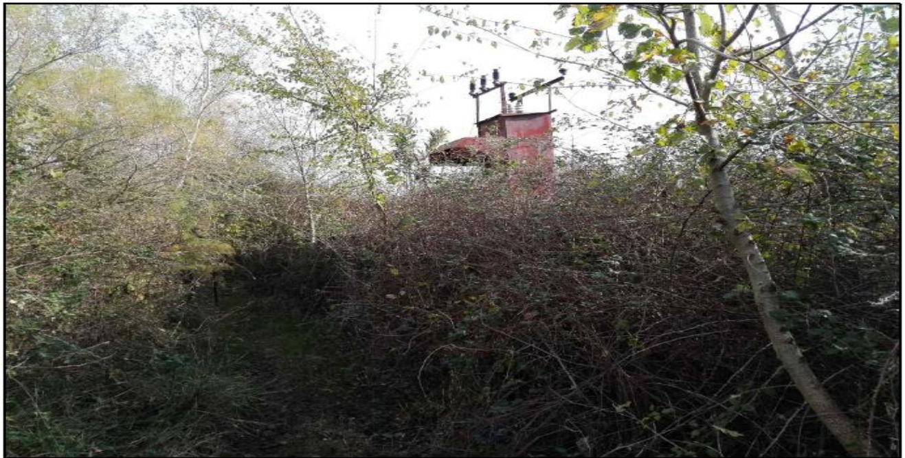
Foto 2: Kabina Metalike-Cerme Shkumbin 01-Fideri Nr.4/10KV-N/St Bicukas-Divjake 35/10KV
