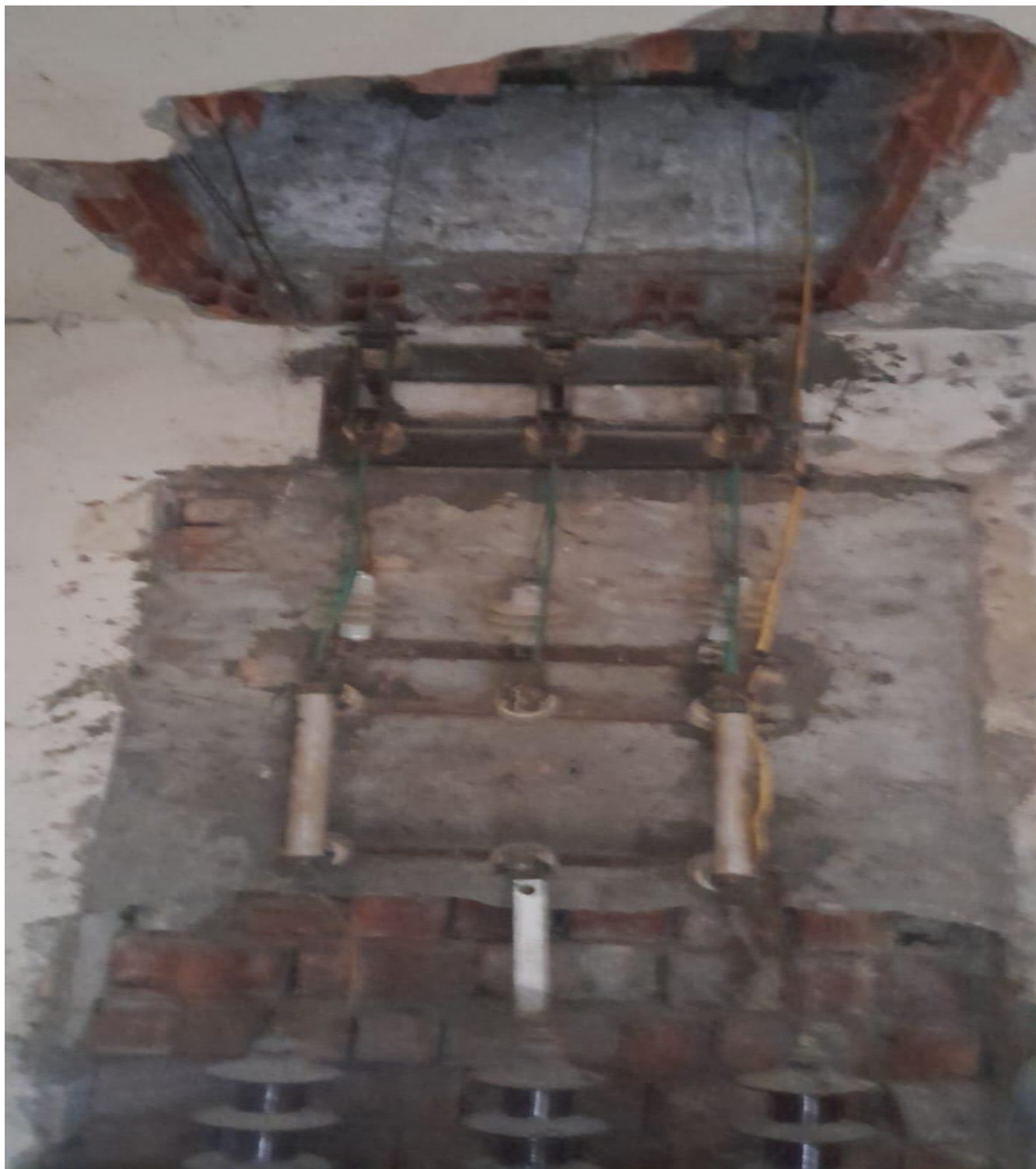
Foto 4: Kabina Murature-Ballagat Qender 03-Fideri Nr.2/10KV-N/St Hyzgjakaj 35/10KV
