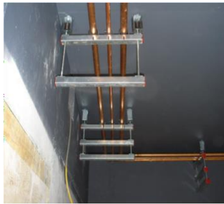
Spring hanger isolation
