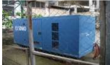
Motogeneratori tip SDMO,me motor John Deere model 6068HF120, 144 kW, i Stacionit te Pompimit te Ujrave te Ndotura
