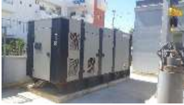
Motogeneratori "TEHNOLINK" me motor Volvo Penta model TAD1642GE, 565 kW ,i Stacionit te Pompimit te Ujrave te Ndotur nr 6,Ksamil
