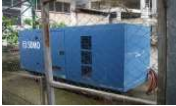
Motogeneratori tip SDMO, me motor John Deere model 6068HF120, 144 kW, i Stacionit te Pompimit te Ujrave te Ndotura
