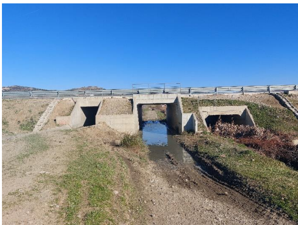
Figura 1-5 C_04, Box Culvert (2m x 2m), Box Underpass(4m x 3m), Box Culvert (4m x 2.5m)
